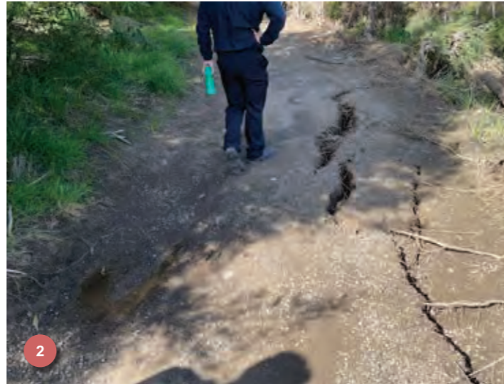
Image: Deep cracks in the regularly inundated area near Crowes Bend
