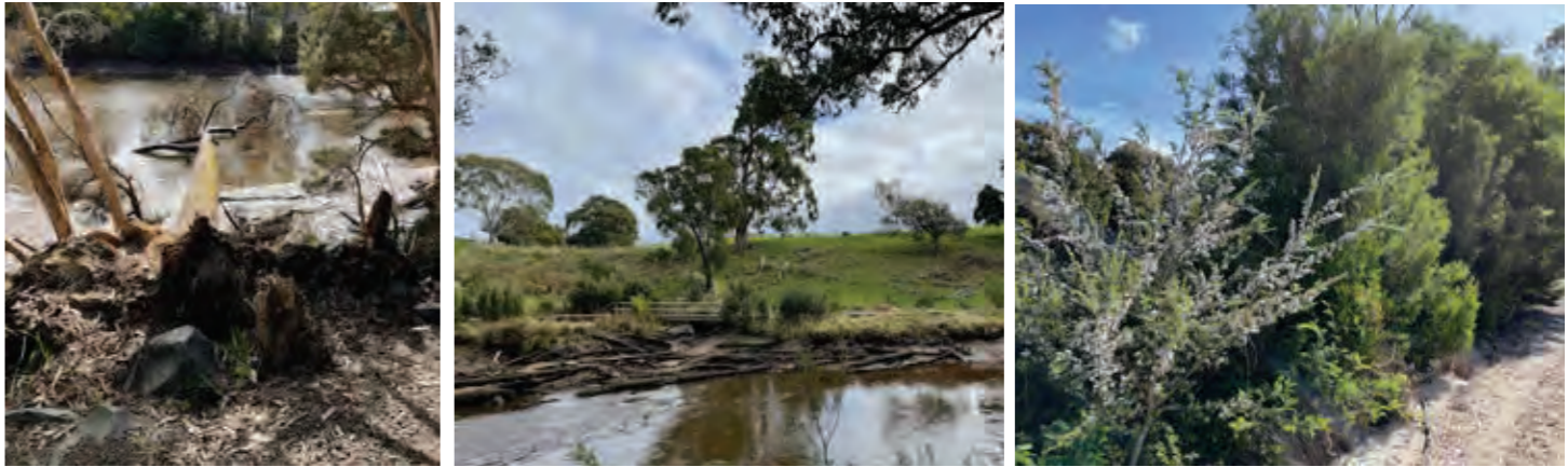
Images: Site photos showing unstable banks along the Inglis River Image: Example of revegetation along bank (near Bass Hwy, south bank)
