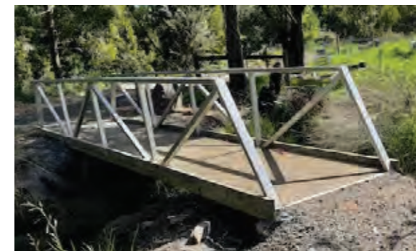
Image at left: Existing metal frame bridge with grating deck, located west of Crows Bend
