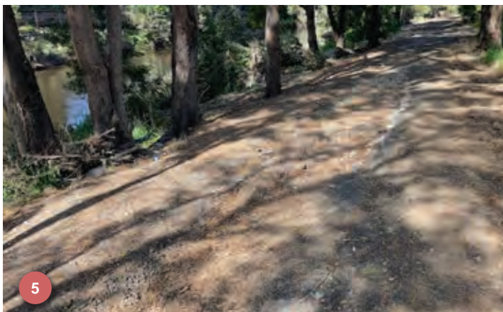
Image: Path washout, south bank near Bass Hwy.
